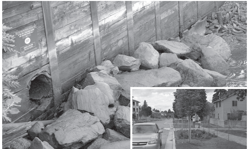
Photo courtesy of the GAIA INSTITUTE Combined sewer outfall at the west end of Schofield Street.
